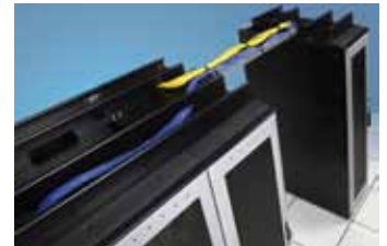
Overhead cable management system
